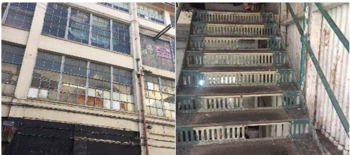
The Leicester Imperial Typewriter Building, where it is estimated that over 50 workplaces are housed. The building is in disrepair and key fire escapes are not fit for purpose.
